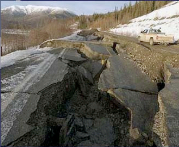
This rupture of the Tok Cutoff Highway in Alaska resulted from a magnitude 7.9 earthquake along the Denali Fault in 2002.
